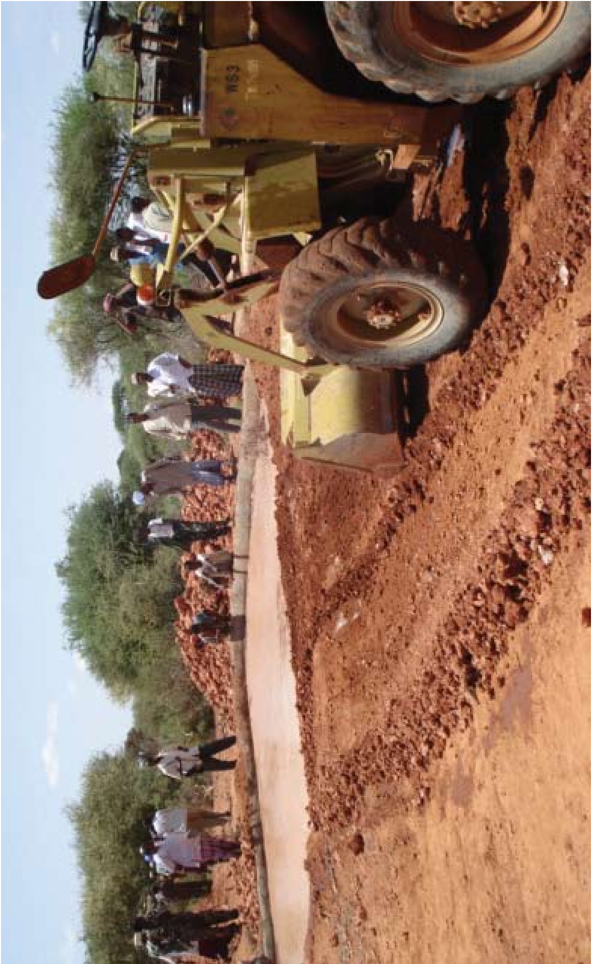
Community elders and officials oversee the destruction of the berkedo (water reservoirs) as agreed as part of the reconciliation process
